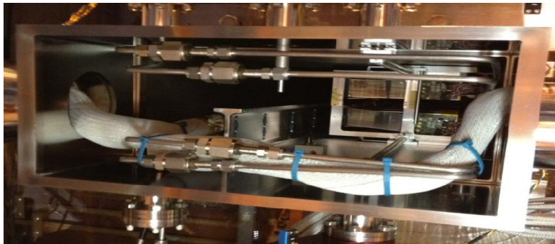
View from upstream looking downstream, through SVT Vac Box Note actual view has more interference with vertical mover rods
