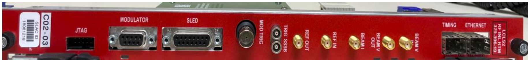
RF Interlock RTM (PC_379_396_19_C02)
