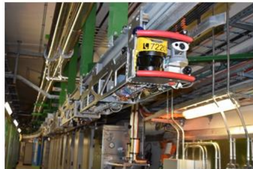
Train Inspection Monorail - TIM
