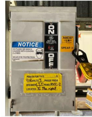
120V Disconnect Switch
