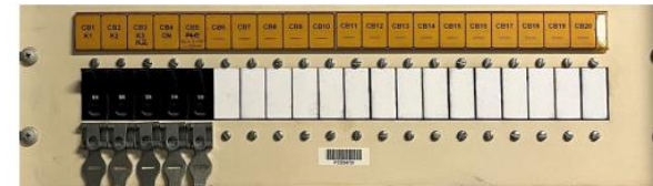
Rack mounted distribution panel
