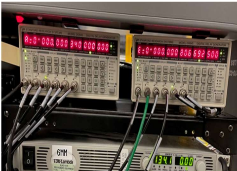
DG645 at eDrive Rack
