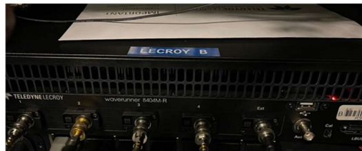
“Lecroy B” Front Panel Power Switch
