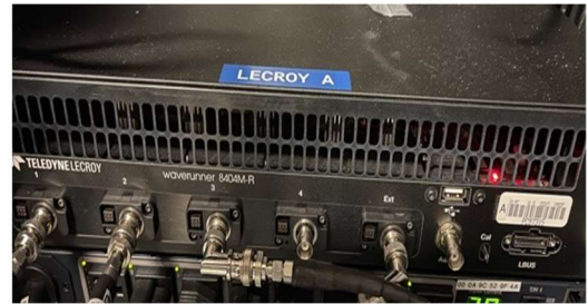
“Lecroy A” Fron Panel Power Switch
