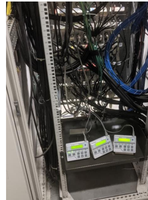
Roughing pump panels @ FKG20-24
