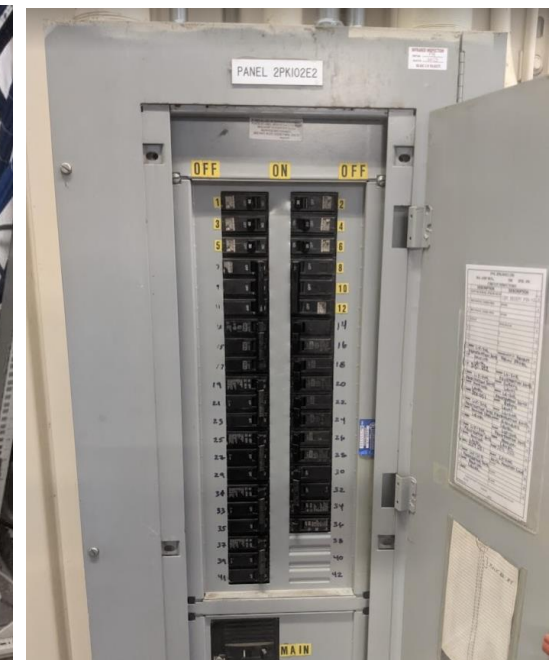
Roughing pump breakers @ 2PK102E2
