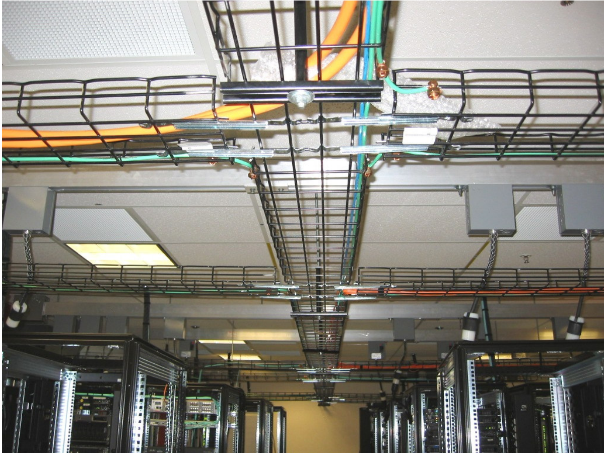
Figure 9. Overhead cable pathways used for routing cables between distribution areas or for ad-hoc cabling between distant racks.
