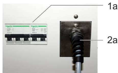
Safety cutouts and mains cable at W80t
