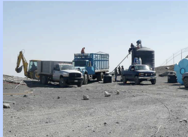
Fig. 3: While the place for the T2 tank is being prepared (left), the water of T3 is being purified.
